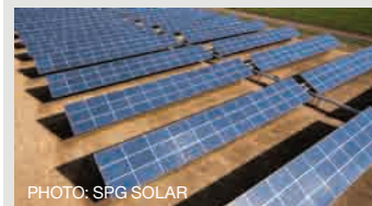
PHOTO: SPG SOLAR
